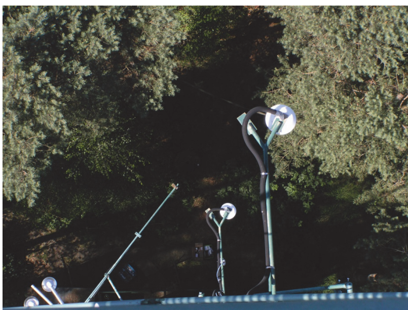
Figure 37 Air is drawn through teflon filter housings covered with a rain shield.
